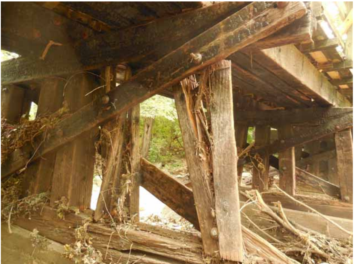
Bridge No. 5 Support Structure Deterioration
