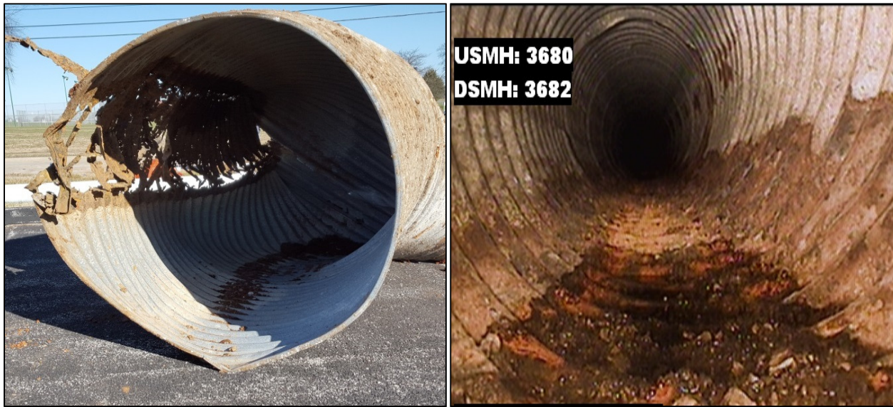
Figure 1. Example of CMP Corrosion and Failure. CMP typically rusts along the bottom of the pipe until the corrosion compromises the structural integrity of the pipe. As a consequence of the corrosion, soil may wash into the pipe causing sink holes to develop or the pipe may collapse causing upstream flooding or pavement failure.
