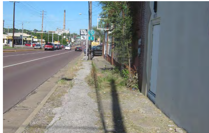
Picture 5. Sidewalk in Poor Condition
