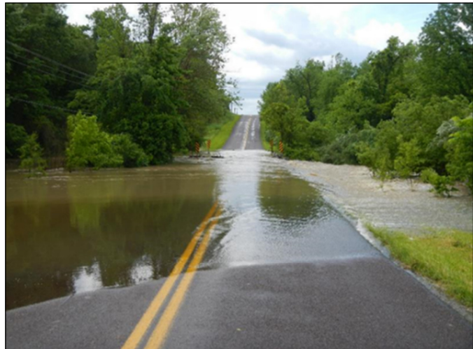
Stormwater system failures contribute to public health, safety, and water quality concerns across Columbia
