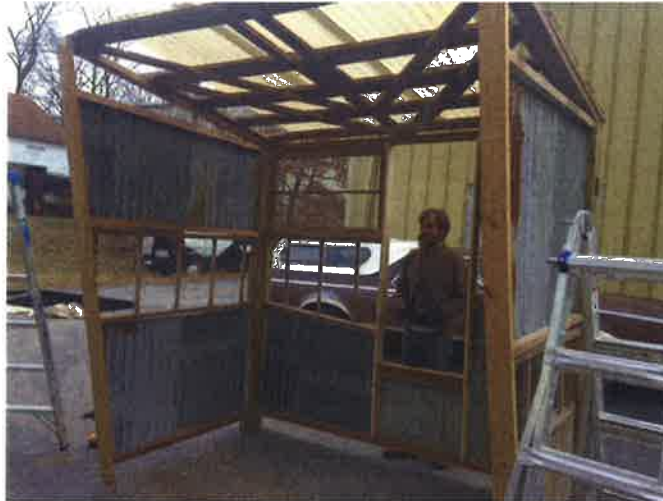
Examples of Bus Shelters installed during T/F 2017
