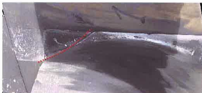
Figure 2: R1 Platform Crack
