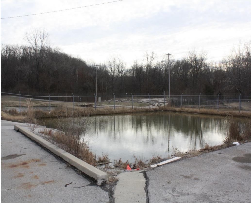
Figure 10 Evaporator pond at Salt Storage Facility
