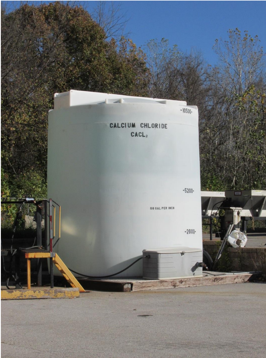
Figure 11 Liquid Calcium Chloride Storage
