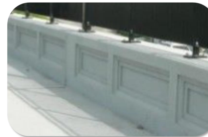
Example of formliner panels on the pedestrian side of the bridge and the highway side of the bridge.
