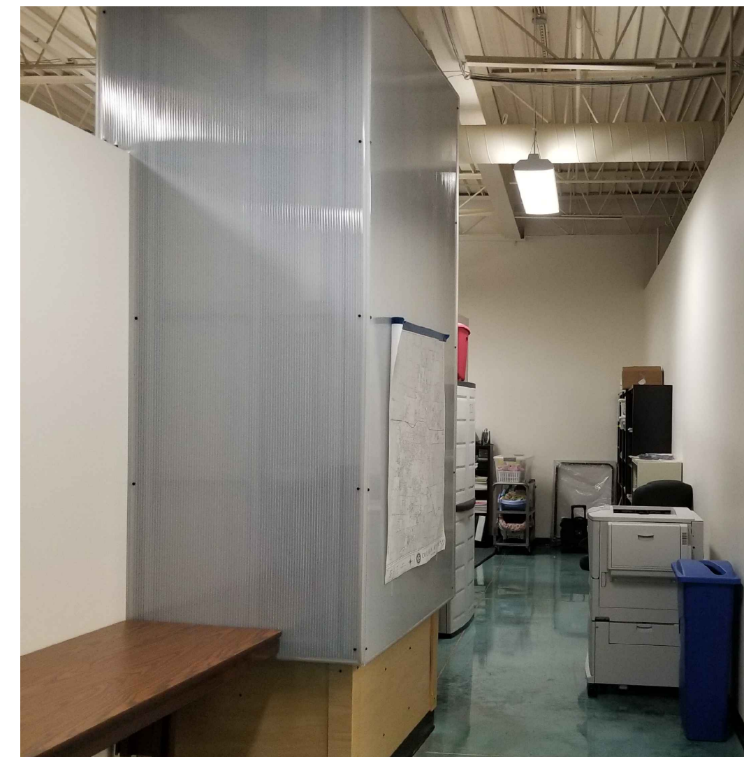
7 EXIST LIGHTBOXES TYP. SCALE: NTS DEMO POLYCARBONATE WALL - INSTALL NEW 5/8" GYP. BD OVER EXIST METAL FRAMING FOR SUSP. CEILING ATTACHMENT
