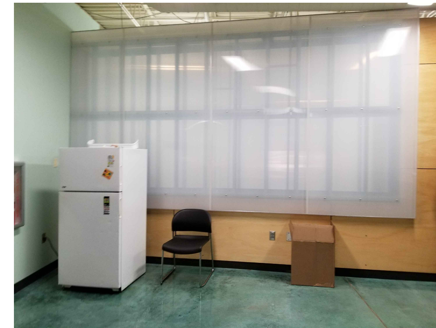
6 EXIST POLYCARBONATE WALL SCALE: NTS DEMO POLYCARBONATE WALL - INSTALL NEW 5/8" GYP. BD OVER EXIST METAL FRAMING FOR SUSP. CEILING ATTACHMENT
