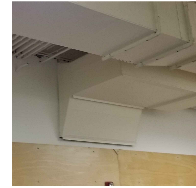
10 EXIST DUCWORK SCALE: NTS MECH. DUCT TO REMAIN - INSTALL NEW 5/8" GYP. BD OVER NEW 3-5/8" METAL FRAMING FOR SUSP. CEILING ATTACHMENT
