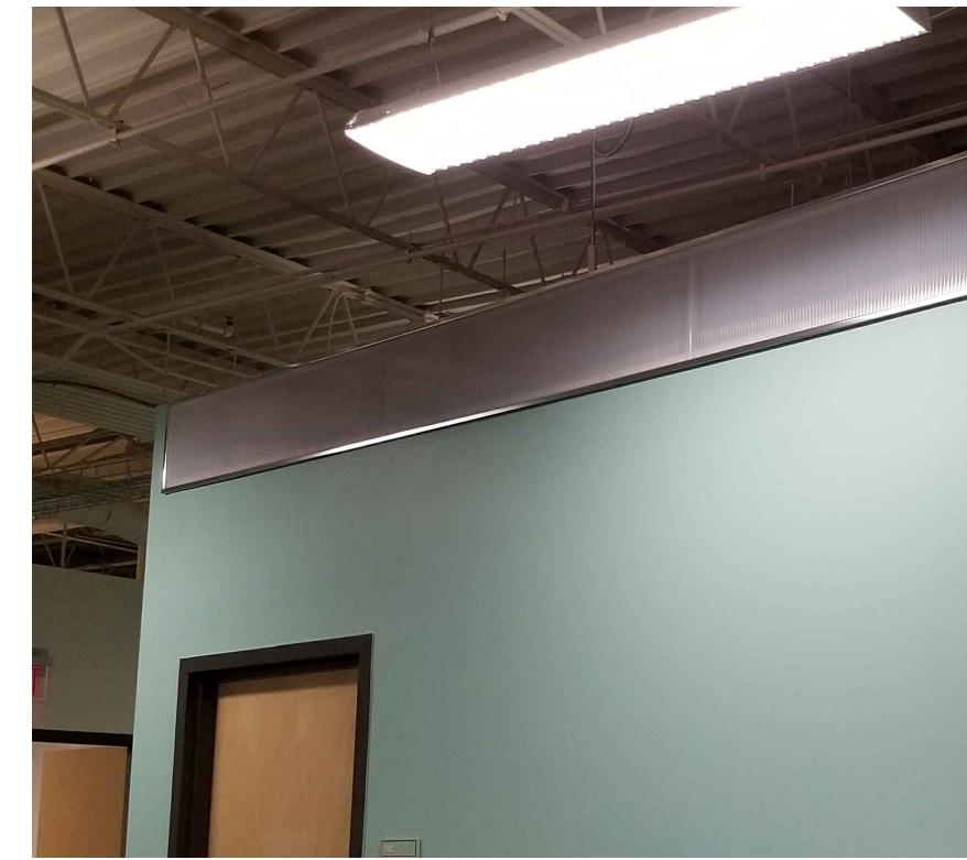
11 EXIST POLYCARBONATE SCALE: NTS DEMO POLYCARBONATE WALL - INSTALL NEW 5/8" GYP. BD OVER EXIST METAL FRAMING FOR SUSP. CEILING ATTACHMENT - SEE 4/44.0
