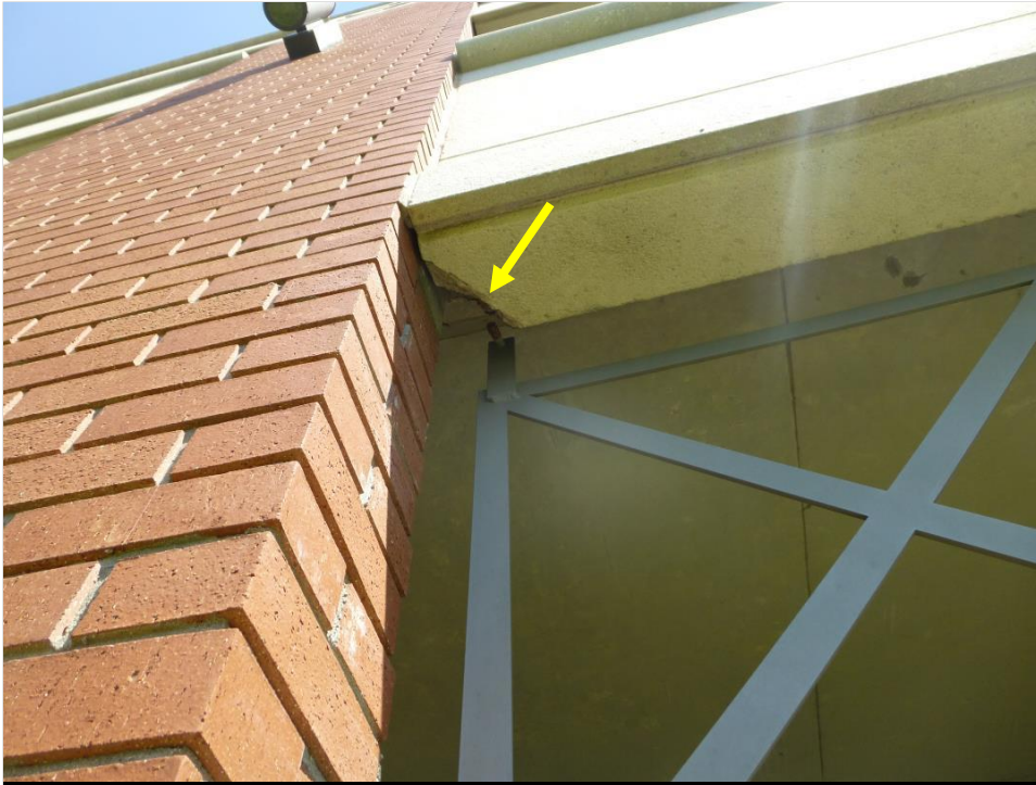
Photo 5 – Spalled façade panel concrete at grill connection.
