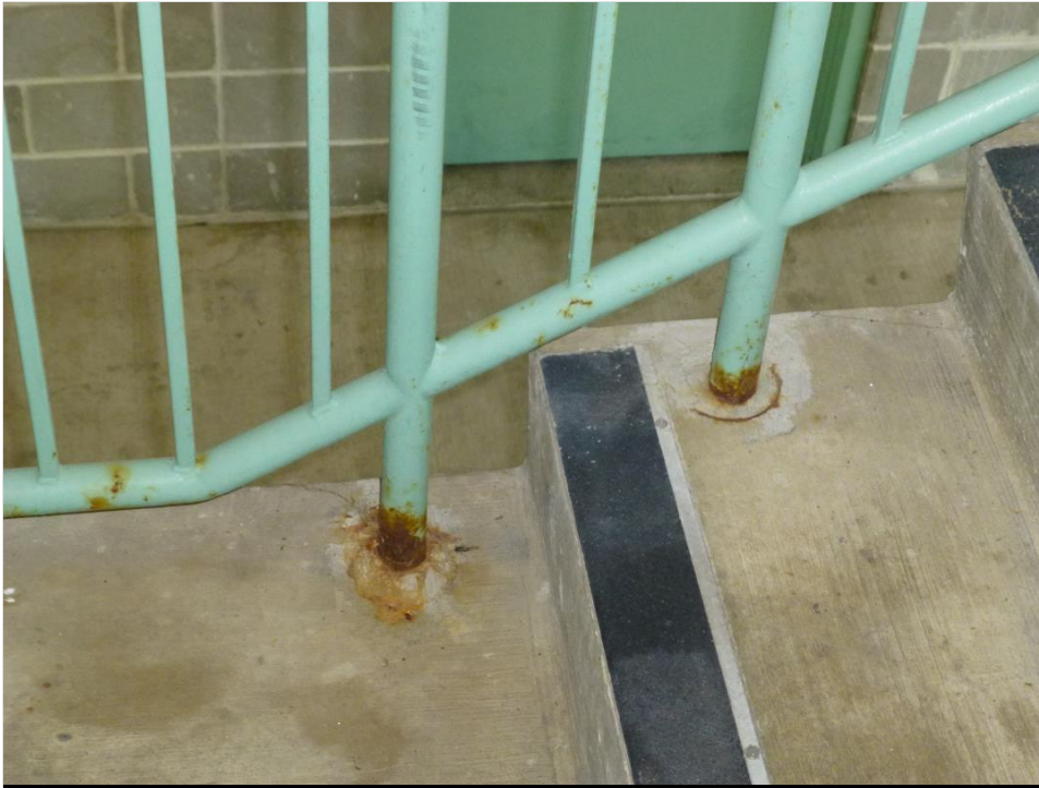
Photo 23 – Surface corrosion at stair handrails and base plate connections.
