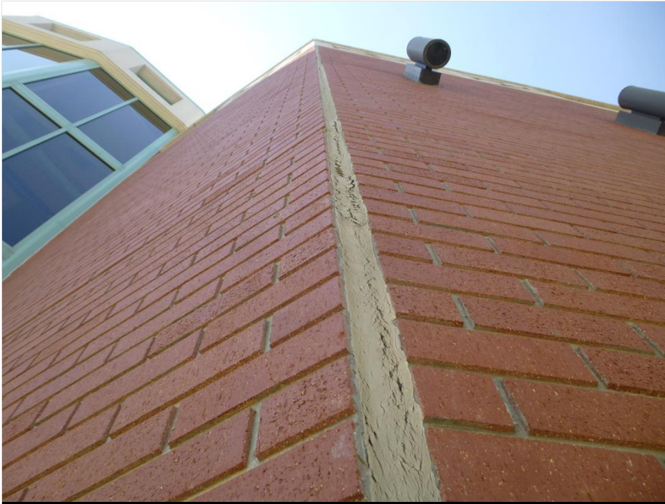
Photo 15 – Close-up of failed sealant at façade isolation joint.
