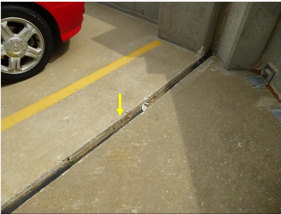
Photo 8 – Adhesion failure observed at Roof Level compression expansion joint.
