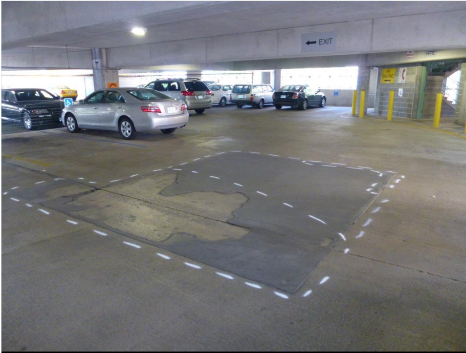
Photo 7 – Spalled and delaminated thin overlay concrete to mitigate water ponding, east elevation entrance.
