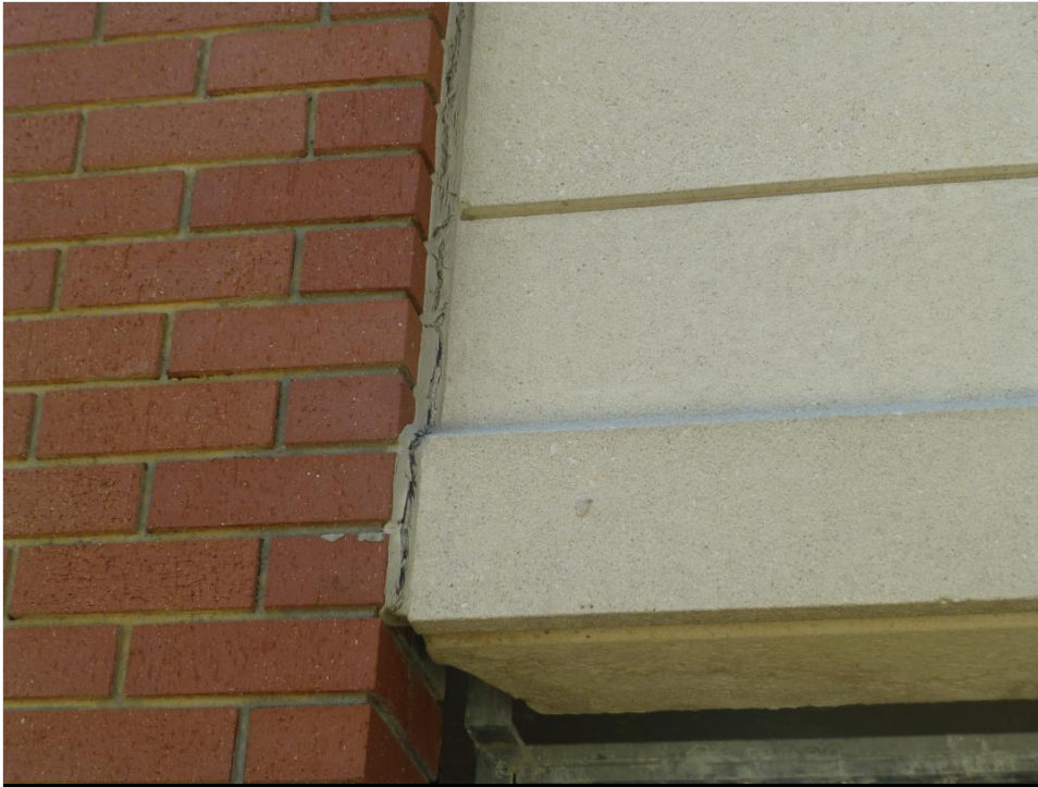
Photo 17 – Close-up of failed sealant between façade panel and brick veneer.
