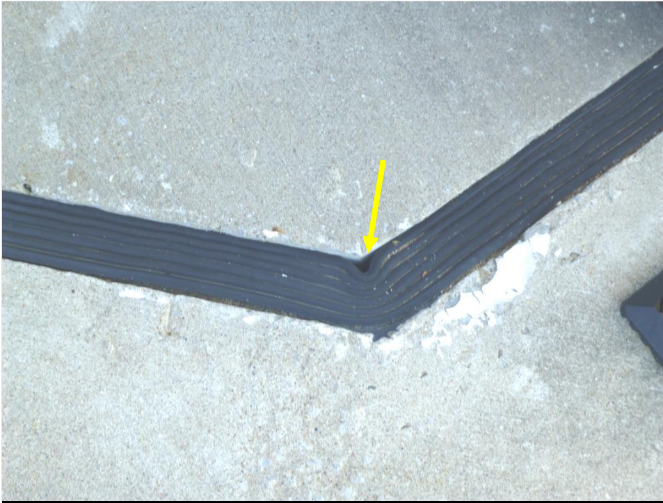
Photo 9 – Opening at compression joint seal.
