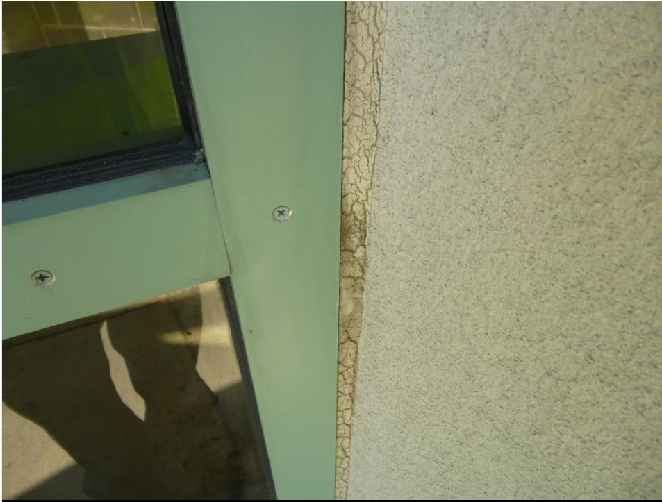
Photo 19 – Failed sealant at window perimeter joints.
