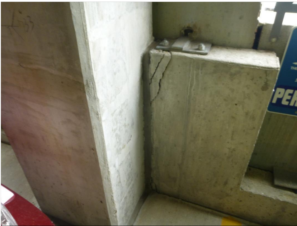
Photo 6 – Cracked and spalled concrete at column-façade panel connection.
