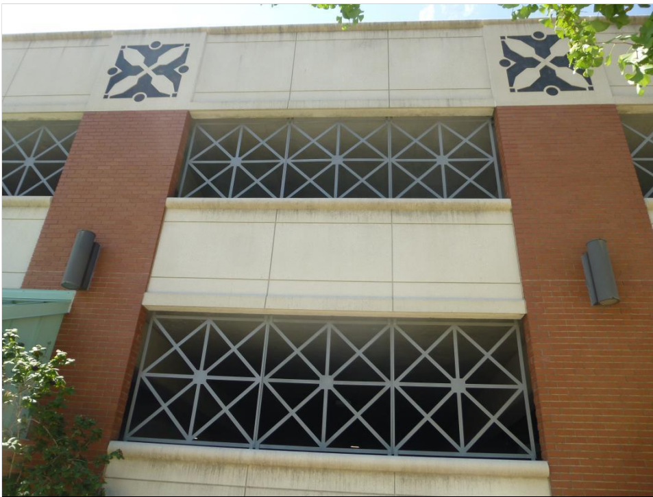
Photo 20 – View of concrete façade panel with embedded dirt and soot.
