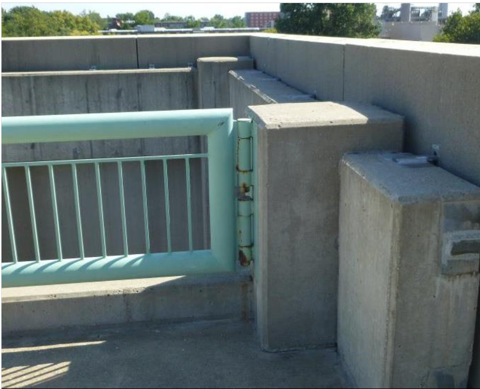
Photo 24 – Surface corrosion at snow-chute gate connection panel.
