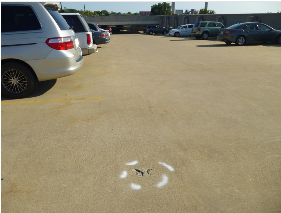
Photo 4 – Isolated area of deteriorated concrete at floor surface, Roof Level.
