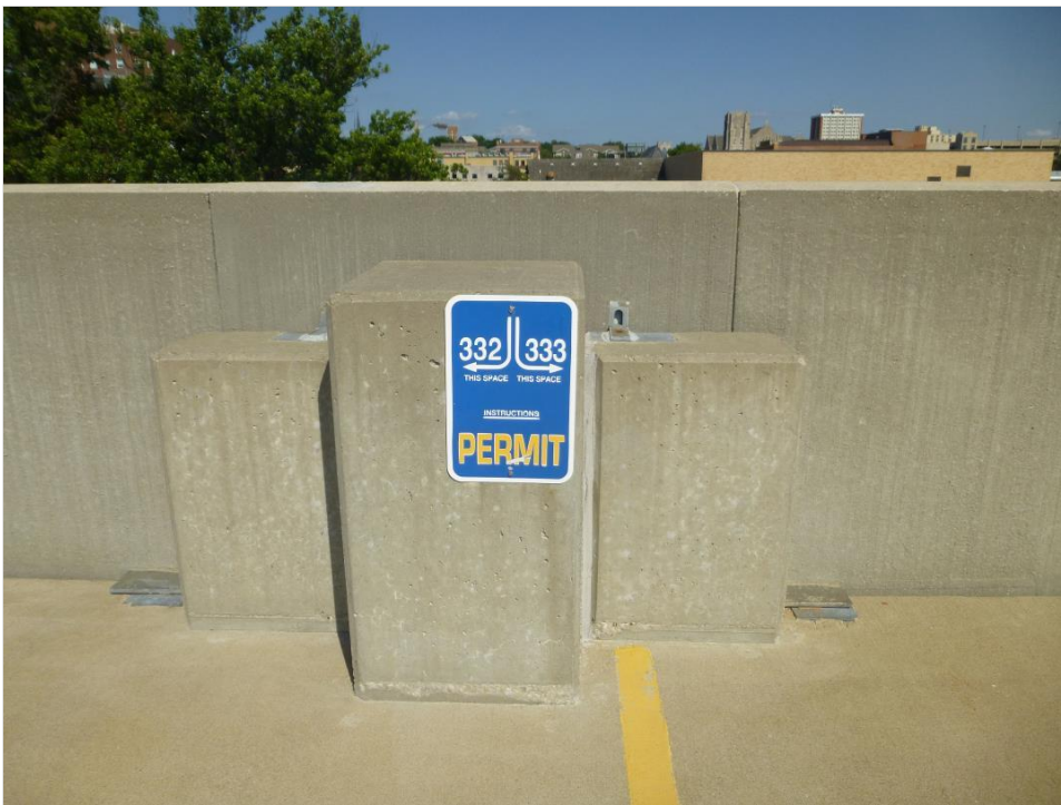
Photo 12 – View of Roof Level stub columns and failed vertical sealant.
