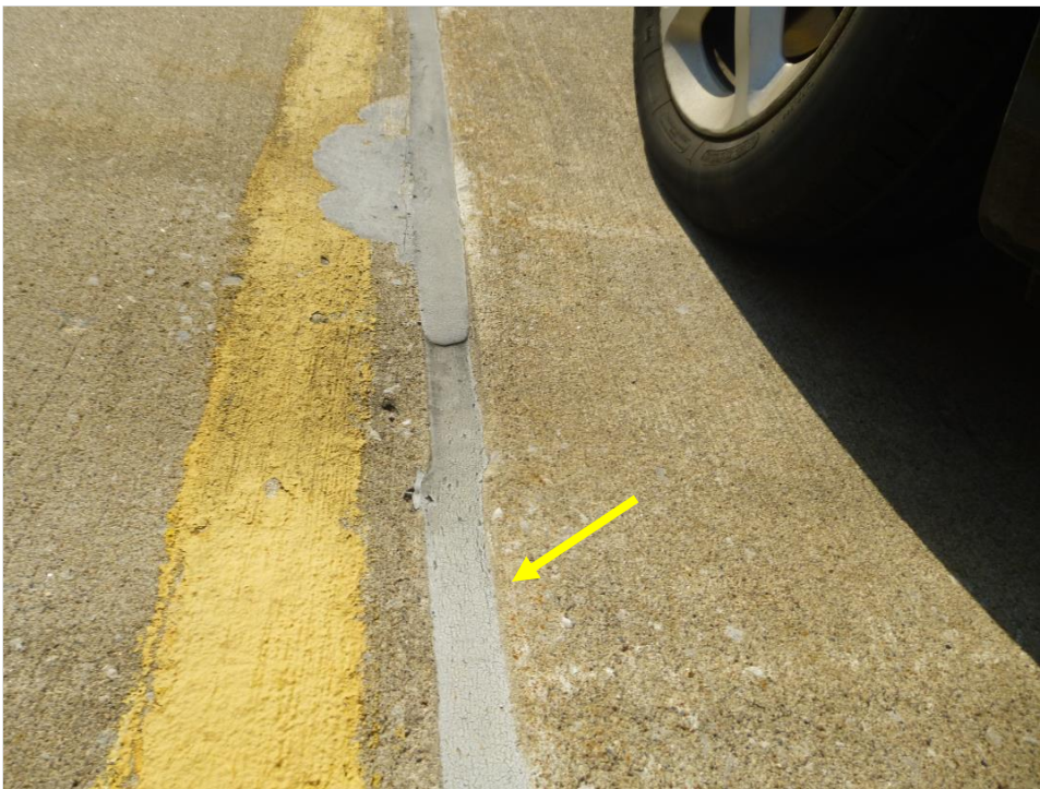
Photo 10 – Alligator cracking observed at control joint.
