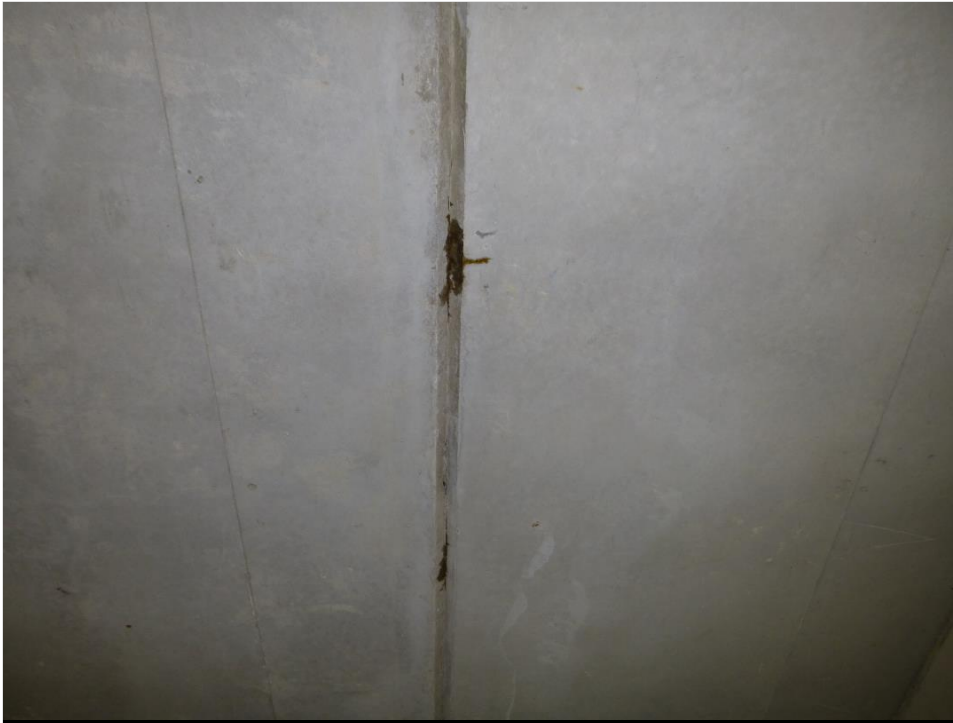
Photo 11 – Water/grease stains on ceiling below control joints.
