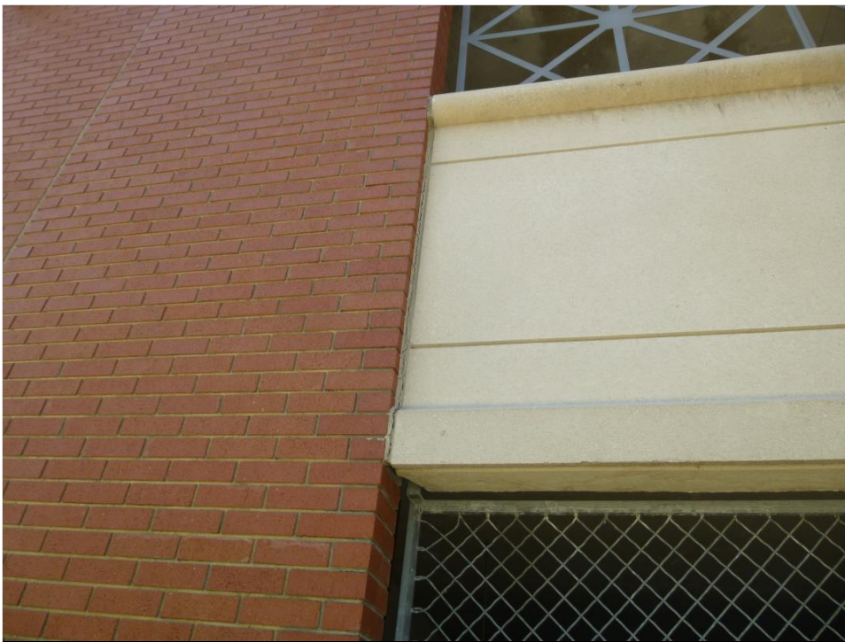
Photo 16 – View of façade panel and failed vertical sealant.
