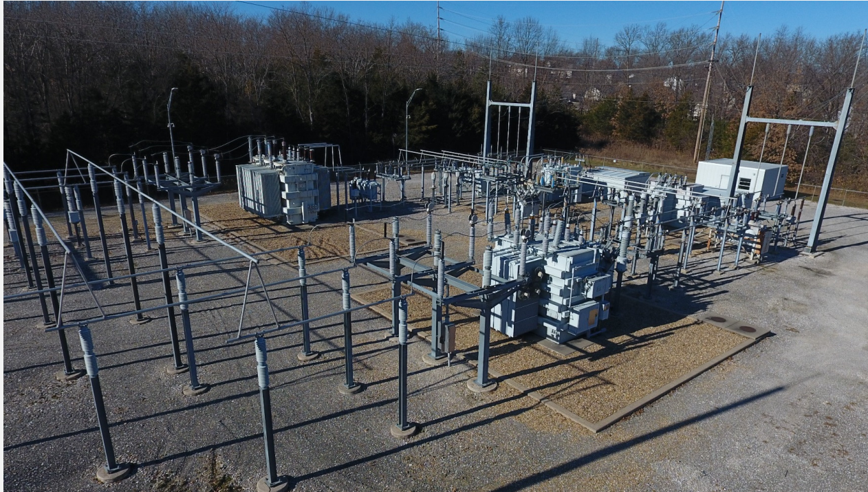
Perche Creek Substation
