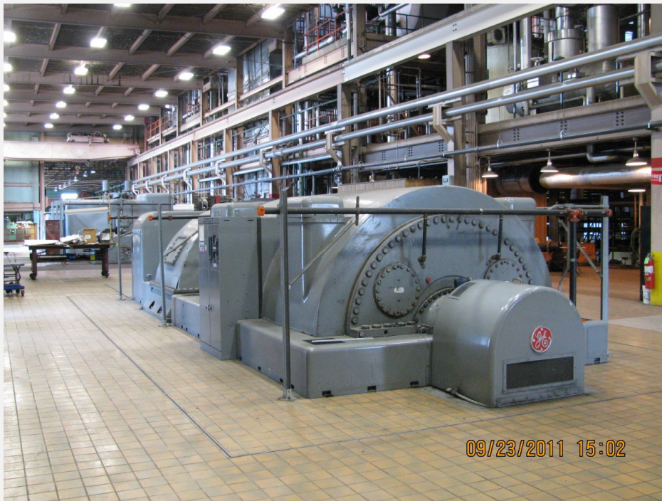
Steam Turbine #8 – 35 MW
