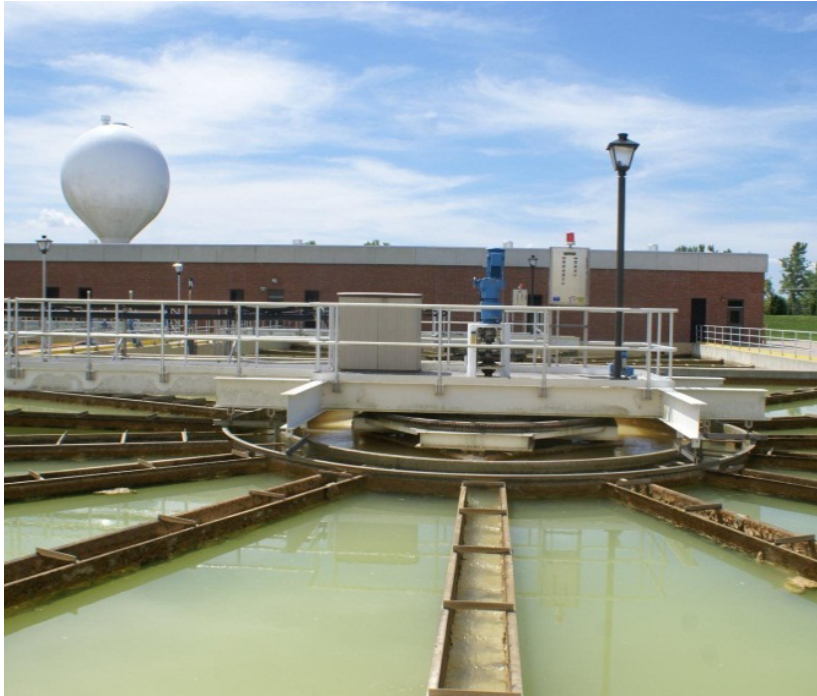
Figure 3-4 McBaine Water Treatment Plant
