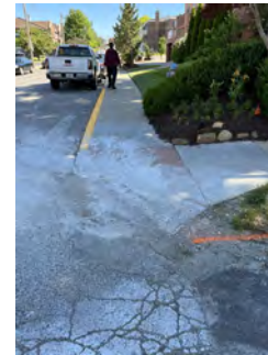
#6: REMOVE & RECONSTRUCT CURB RAMP & 1 SIDEWALK PANEL EAST SIDE/2 SIDEWALK PANELS NORTH SIDE, TO CREATE LANDING & RAMPS. REMOVE & RECONSTRUCT CURB & GUTTER. INSTALL DETECTABLE WARNING.
