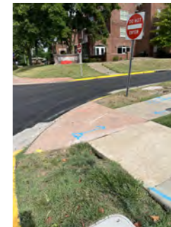
#5: REMOVE & RECONSTRUCT CURB RAMP & 1 SIDEWALK PANEL ON EACH SIDE TO CREATE LANDING & RAMPS. REMOVE & RECONSTRUCT CURB & GUTTER. INSTALL DETECTABLE WARNING.
