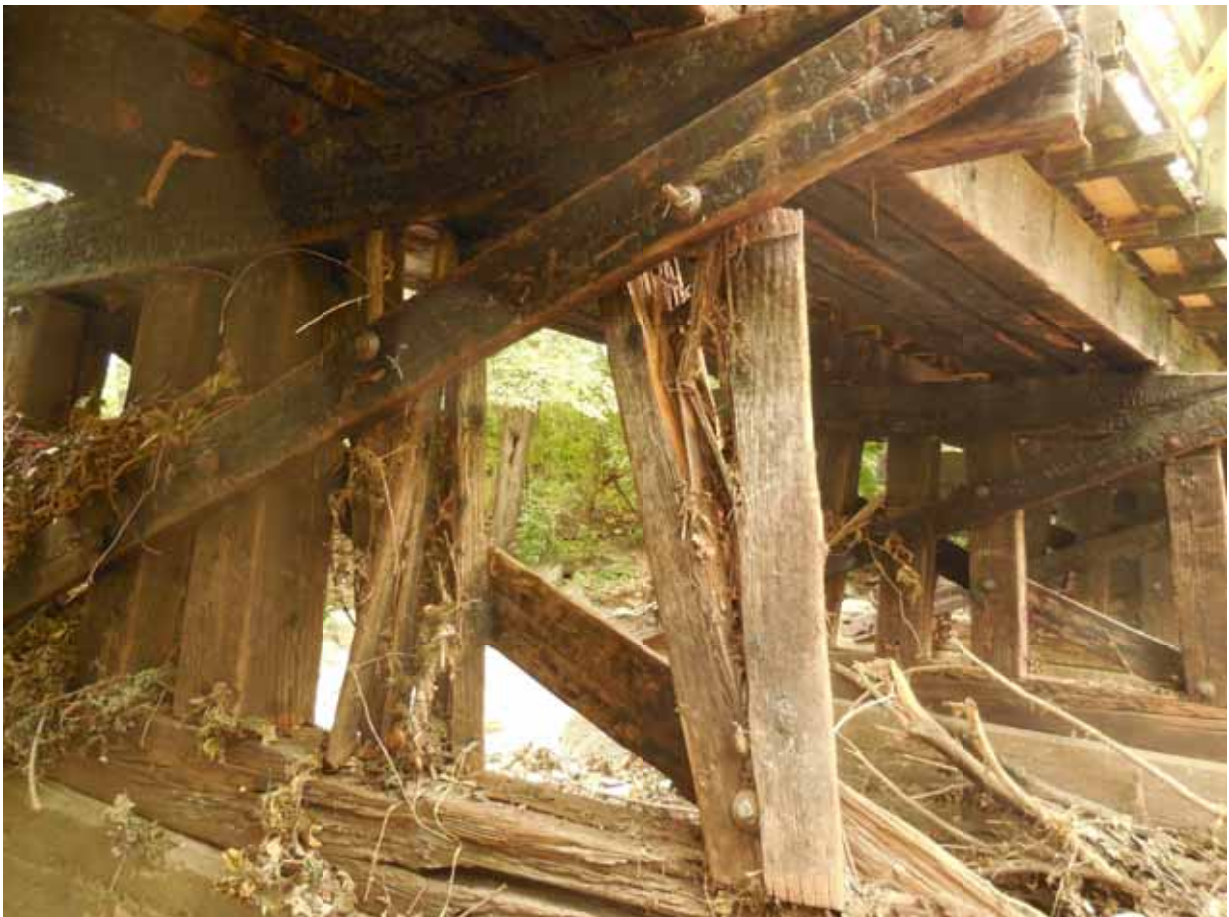
Bridge No. 5 Support Structure Deterioration
