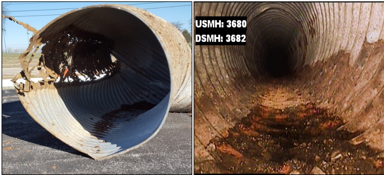
Figure 1. Example of CMP Corrosion and Failure. CMP typically rusts along the bottom of the pipe until the corrosion compromises the structural integrity of the pipe. As a consequence of the corrosion, soil may wash into the pipe causing sink holes to develop or the pipe may collapse causing upstream flooding or pavement failure.
