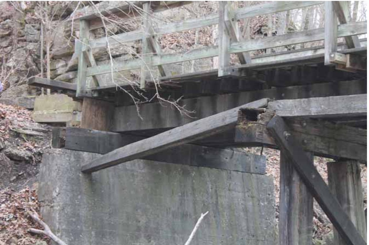
Bridge No. 7 Support Structure Deterioration
