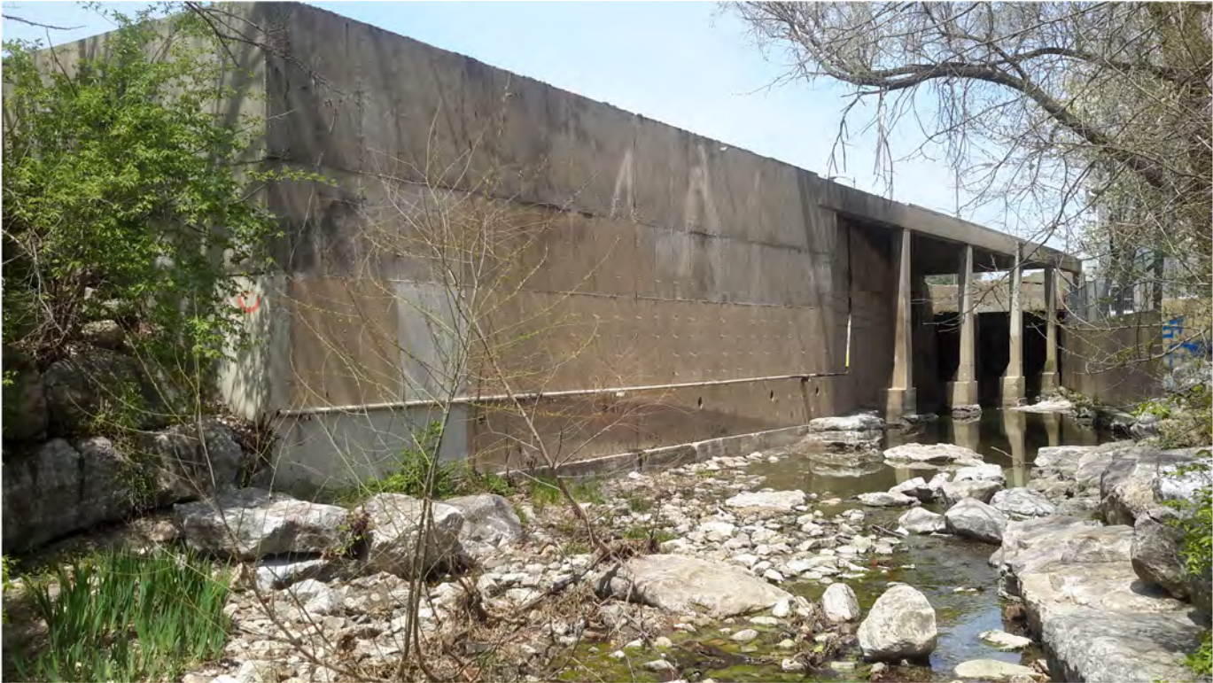
View from Flat Branch Park toward McAdams retaining wall (future creek restoration area)
