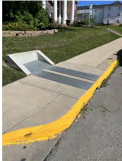
#1: REMOVE TRENCH GRATES IN SIDEWALK & REPLACE WITH NEENAH R-4999-DX WITH TYPE D LID TO REMOVE SLIP HAZARD. SEE DETAIL ON SHEET 3.
