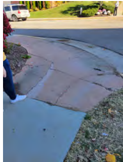
#5: REMOVE & RECONSTRUCT CURB RAMP & NORTH SIDE SIDEWALK PANELS TO CREATE SMALLER LANDING & RAMPS. REMOVE & RECONSTRUCT CURB & GUTTER. INSTALL DETECTABLE WARNING.
