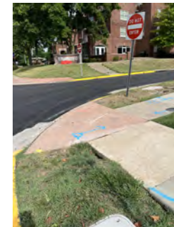
#5: REMOVE & RECONSTRUCT CURB RAMP & 1 SIDEWALK PANEL ON EACH SIDE TO CREATE LANDING & RAMPS. REMOVE & RECONSTRUCT CURB & GUTTER. INSTALL DETECTABLE WARNING.
