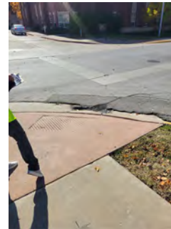
#4: REMOVE & RECONSTRUCT CURB RAMP & 2 SIDEWALK PANEL ON EACH SIDE TO CREATE LANDING & RAMPS. REMOVE & RECONSTRUCT CURB & GUTTER. INSTALL DETECTABLE WARNING. SEE SHEET 11.
