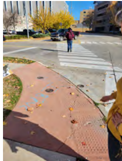
#7: REMOVE & RECONSTRUCT CURB RAMP & 1 SIDEWALK PANEL ON EACH SIDE TO CREATE LANDING & RAMPS. REMOVE & RECONSTRUCT CURB & GUTTER. INSTALL DETECTABLE WARNING.
