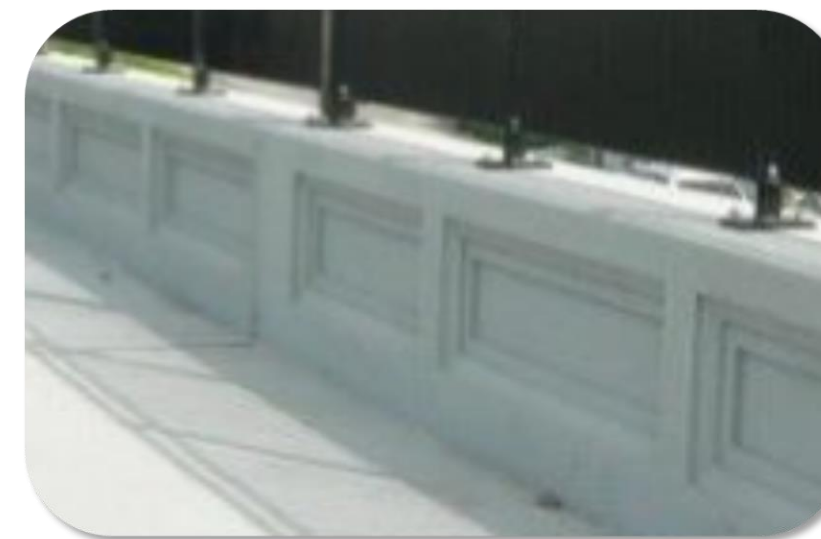
Example of formliner panels on the pedestrian side of the bridge (on this project, the panels will be on the outside of the bridge. Refer to image above for panel spacing with fence posts.
