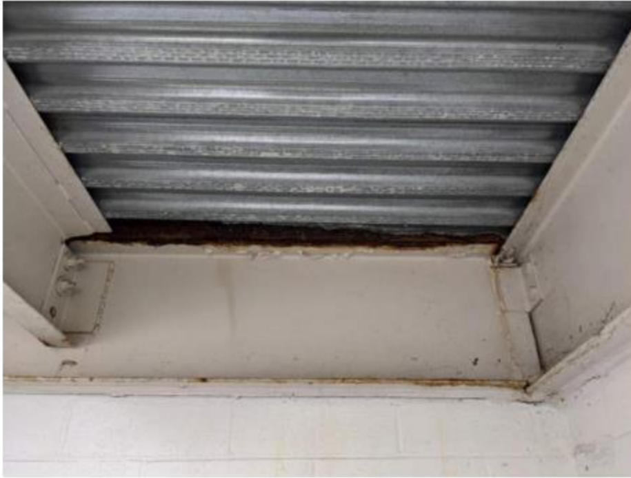
8&C -Photo 111. Typical corrosion on underside of southwest stair tower landings.
