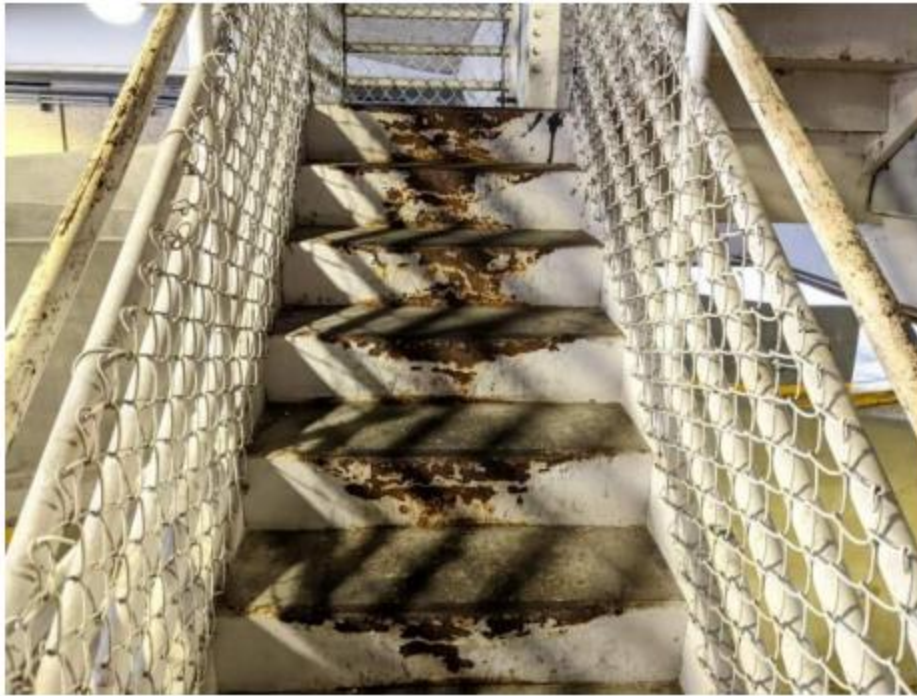
8&C -Photo 109. Interior stair tower with moderate to severe corrosion.
