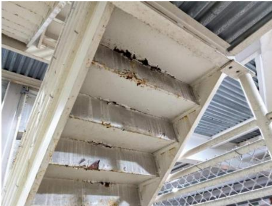
8&C -Photo 110. Underside of interior stair tower with moderate to severe corrosion.
