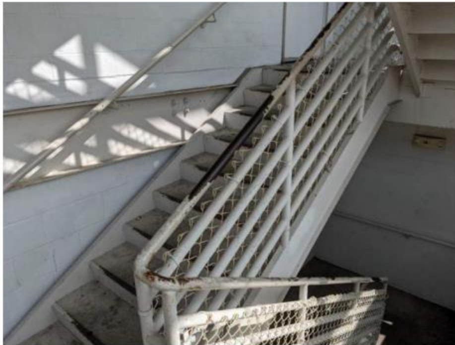
8&C -Photo 112. Typical worn paint on stair tower railings.
