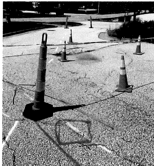
Settling of pavement, crater-shape.
