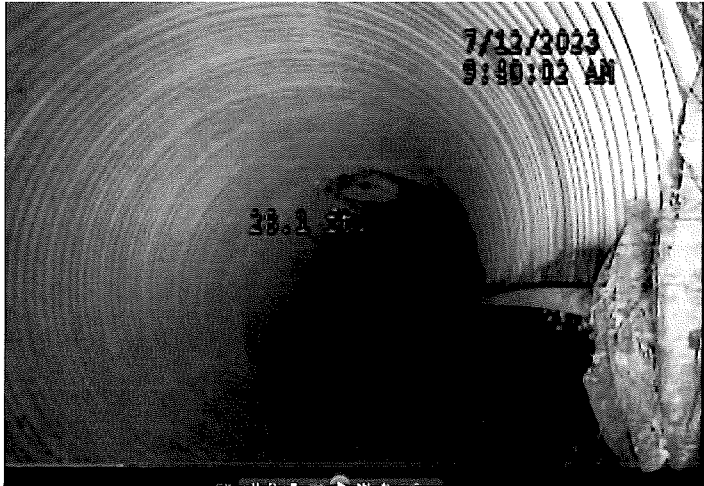
Boring rod, tip abandoned in storm pipe.
