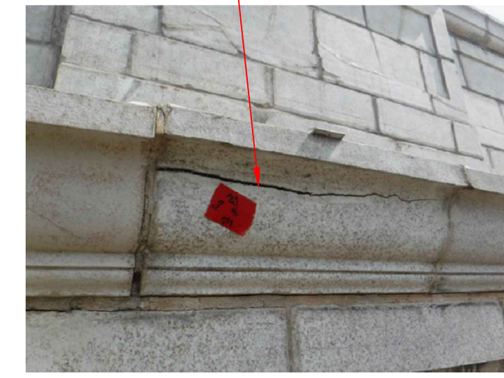
RI 5. REPLACE EXISTING TC CRACK SEALANT AND PROVIDE SEALANT AT UNSEALED TC UNIT CRACKS.
