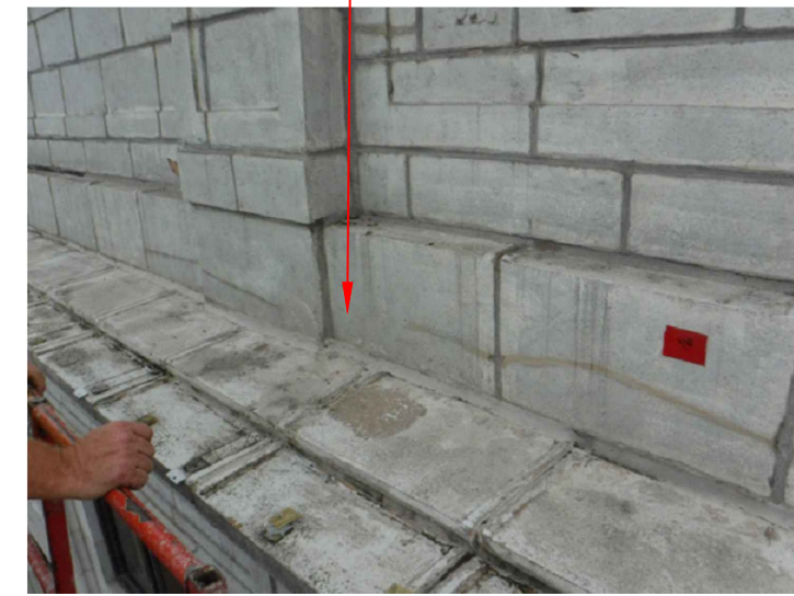
RI 1. REPLACE FAILED TERRA COTTA COLOR COATINGS AND GLAZE.
