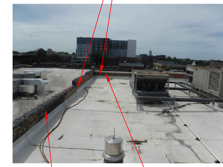
RI 8. REPOINT TC ISOLATED MORTAR JOINTS AT MASONRY BELOW THE CORNICE AND THE BACKSIDE OF THE PARAPET WALLS AND PARTY WALL. RI 11. PARAPET WALL BACKSIDE AND PARTY WALL MASONRY WATER REPELLENT APPLICATION.
