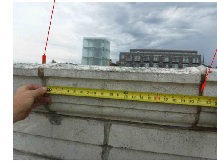
RI 4. REPLACE TC UNIT JOINT MORTAR/SEALANT AT 100-PERCENT OF THE TC UNIT SKYVIEW SURFACES AS INDICATED ON THE DRAWINGS.
