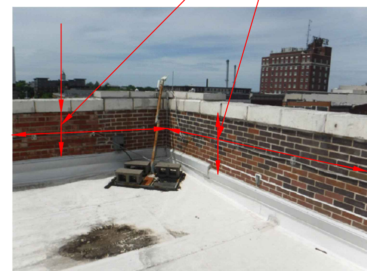
RI 8. REPOINT TC ISOLATED MORTAR JOINTS AT MASONRY BELOW THE CORNICE AND THE BACKSIDE OF THE PARAPET WALLS AND PARTY WALL. RI 11. PARAPET WALL BACKSIDE AND PARTY WALL MASONRY WATER REPELLENT APPLICATION.
