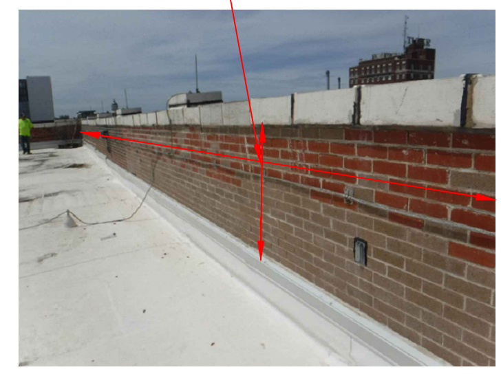
RI 8. REPOINT TC ISOLATED MORTAR JOINTS AT MASONRY BELOW THE CORNICE AND THE BACKSIDE OF THE PARAPET WALLS AND PARTY WALL. RI 11. PARAPET WALL BACKSIDE AND PARTY WALL MASONRY WATER REPELLENT APPLICATION.
