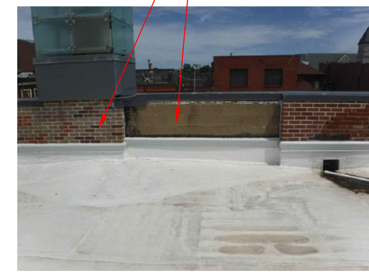
RI 8. REPOINT TC ISOLATED MORTAR JOINTS AT MASONRY BELOW THE CORNICE AND THE BACKSIDE OF THE PARAPET WALLS AND PARTY WALL. RI 11. PARAPET WALL BACKSIDE AND PARTY WALL MASONRY WATER REPELLENT APPLICATION.
