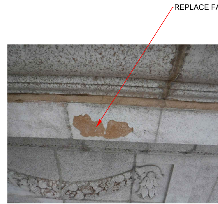
RI 1. REPLACE FAILED TERRA COTTA COLOR COATINGS AND GLAZE.
