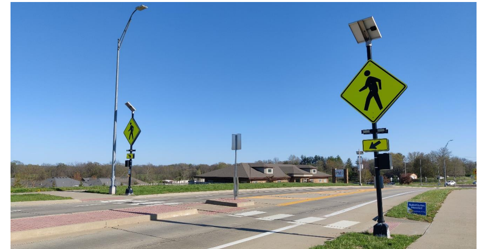
Scott Blvd South of Abbington Terrace (RRFB)
