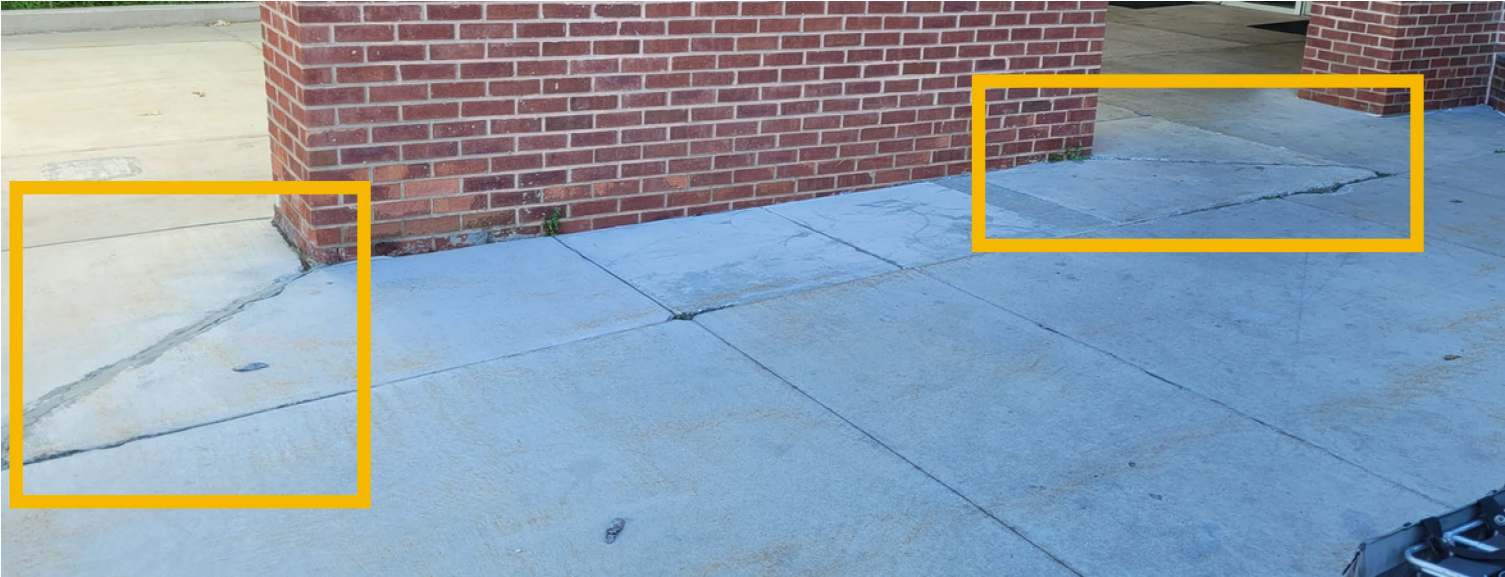
ARC Entry Area
