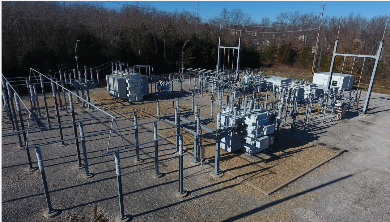
Perche Creek Substation
