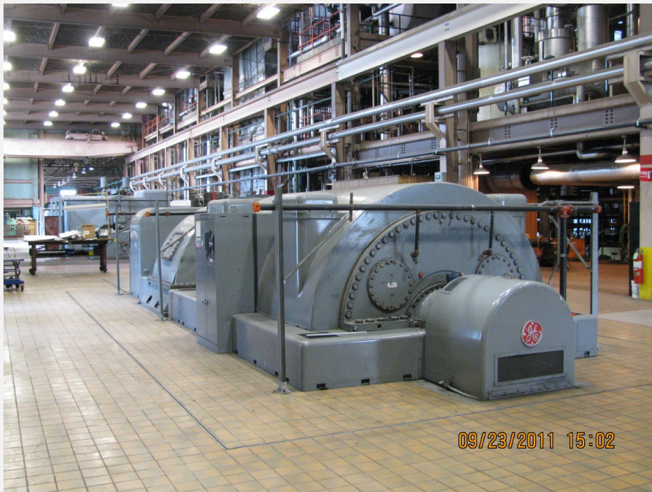
Steam Turbine #8 – 35 MW
