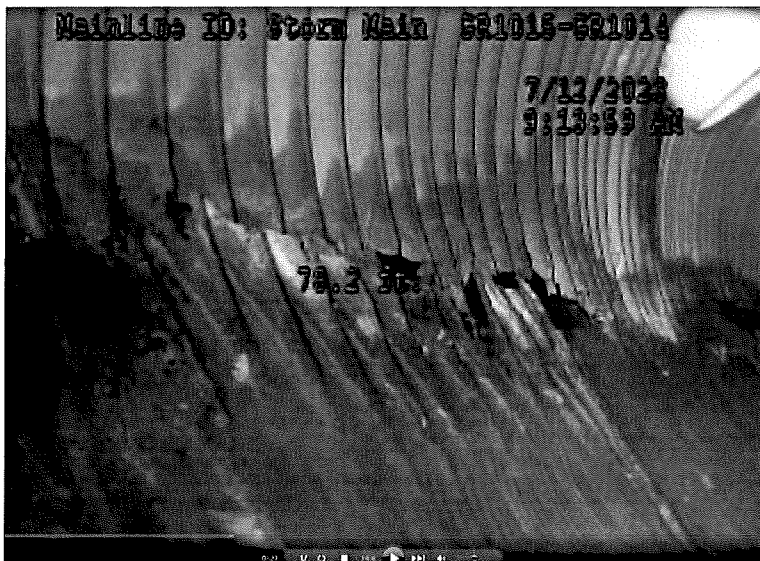
Pipe flowline is corroded and washed away. Bare soil exposed.
