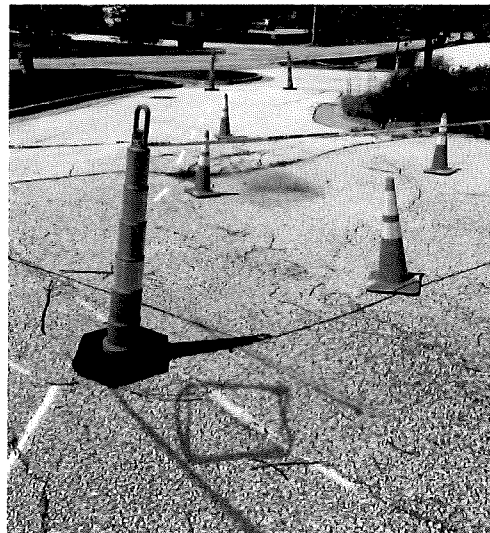
Settling of pavement, crater-shape.
