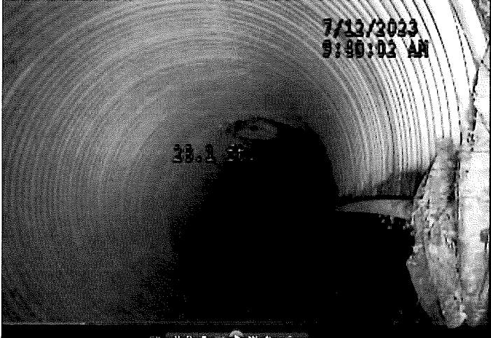
Boring rod, tip abandoned in storm pipe.
