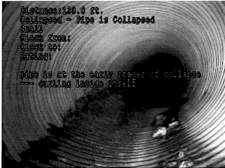
Pipe at early stages of collapse. Significant deformation, some of the pipe flowline is corroded.
